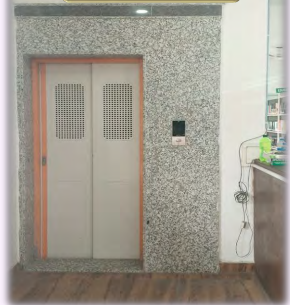
Lift Facility in Library Building
